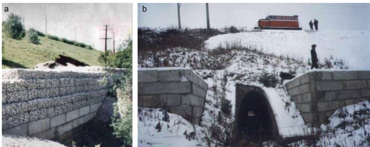
Picture 2 The mechanical-stabilized earth walls on Gorkovskaya Railway a) with gabions on top б) with concrete blocks (photo Vinogradov V.V.)
