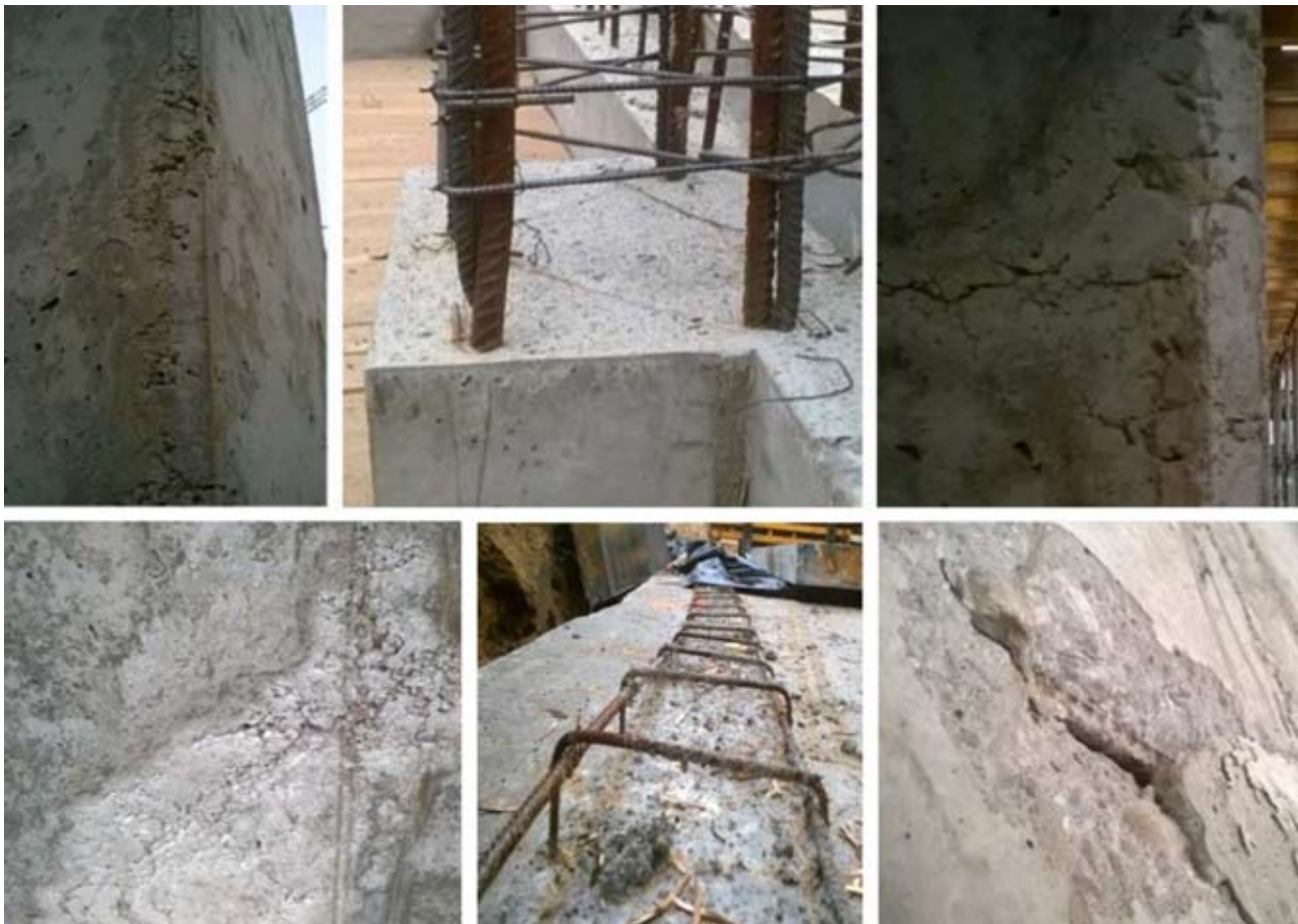
Figure 5. Bad quality of reinforced concrete elements.
